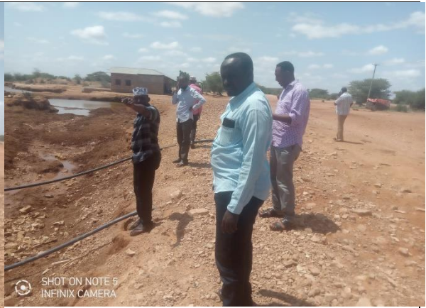
Damaged water pipes at Gingo village in Khalalio
