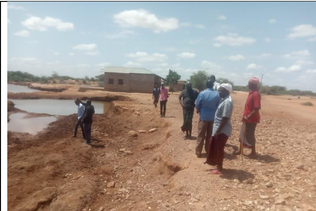
Technical team and local community assessing a section of damaged road at Gingo village
